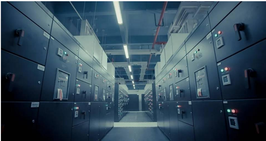
Comac Shanghai Data Center
