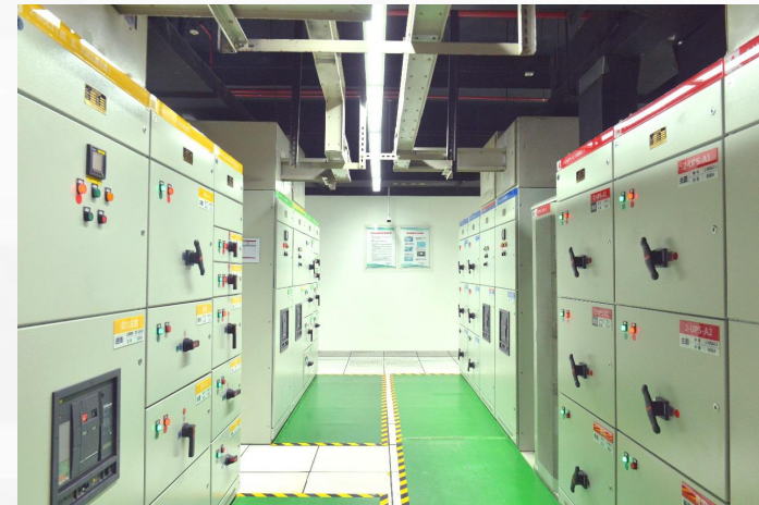
CCC Cloud Data Center
