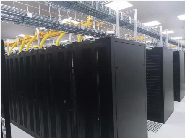
State Grid Zhejiang Data Center
