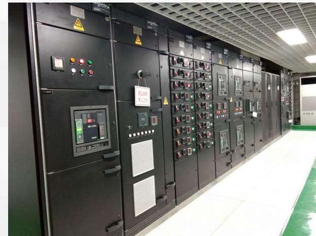
Jiangxi Provincial Info. Center Data Center
