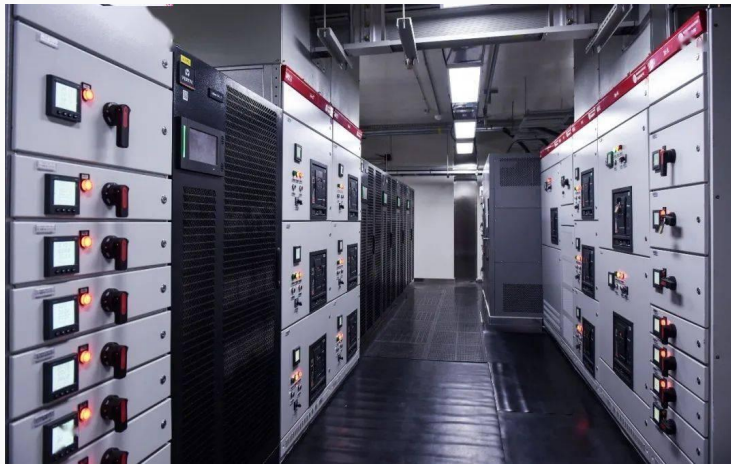
China Unicom Changsha Data Center
