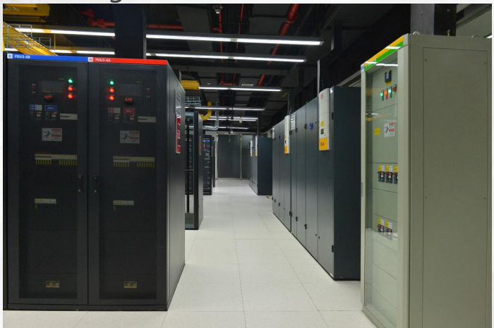
China Zheshang Bank Data Center
